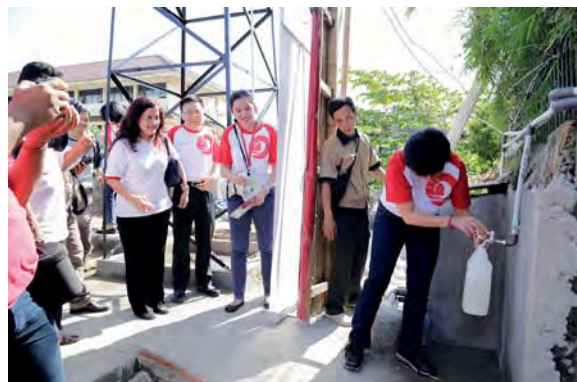
Pengecekan hasil instalasi air bersih di Kali Adem Testing clean water at Kali Adem
