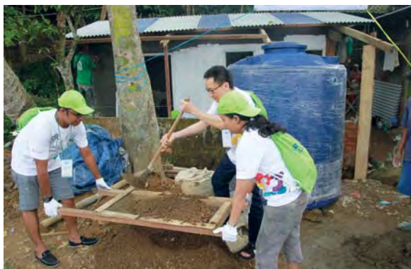
Pembangunan instalasi air bersih, Desa Ciaseupan Bogor Building clean water installation, Ciaseupan Village Bogor
